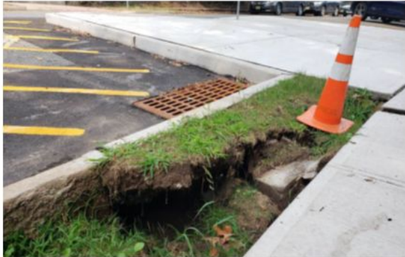
Sinkhole at Dunnell Road near Memorial Park and Maplewood Train Station
