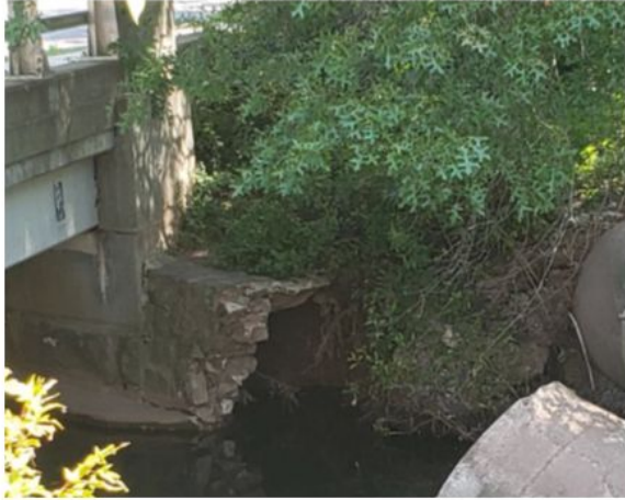
Stream Erosion and Undermining at Oakland Road
