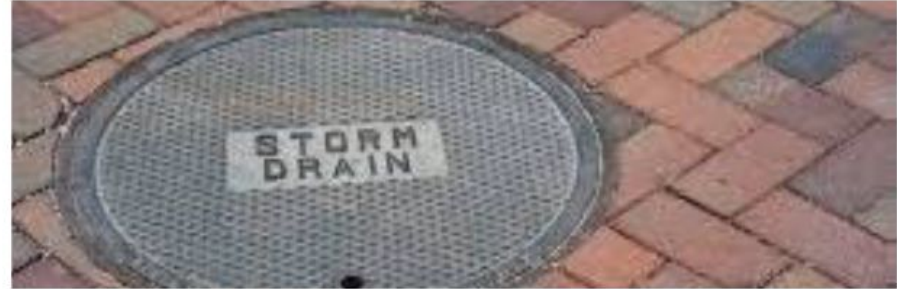
839 Storm Maintenance Holes
