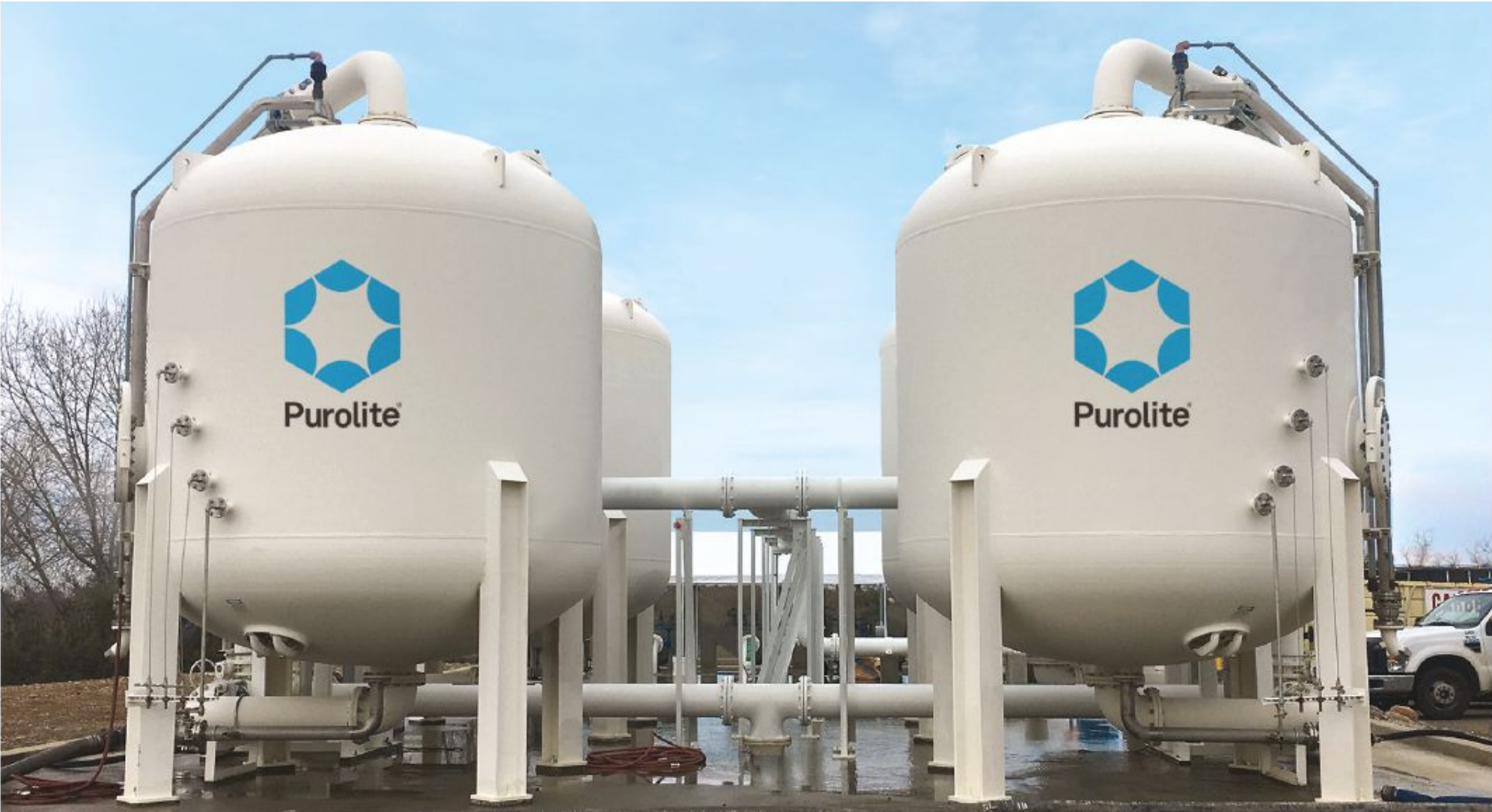
Ion Exchange Vessels
