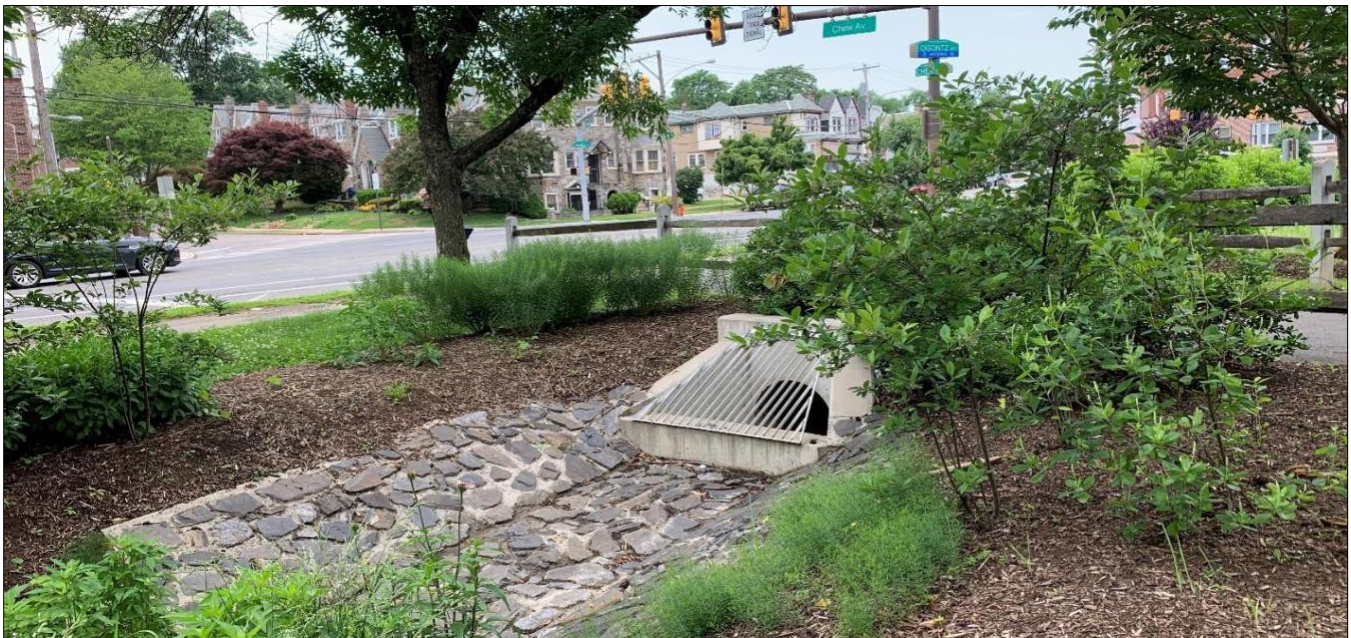
Figure 4. Kemble Park bioswale with trash rack and riprap in Philadelphia, PA. Credit: E&LP, Inc.
